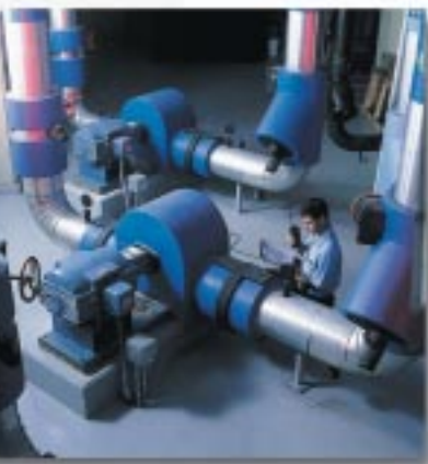
Traditional pump room application for VFDs
